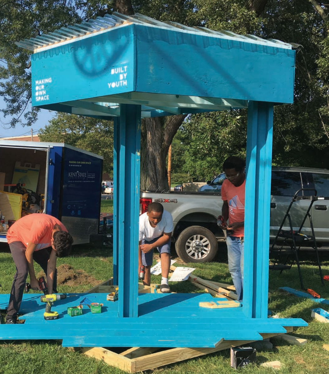
BELOW E.J., Jaleel, and Ben working on the Lakeview Road bus shelter.
